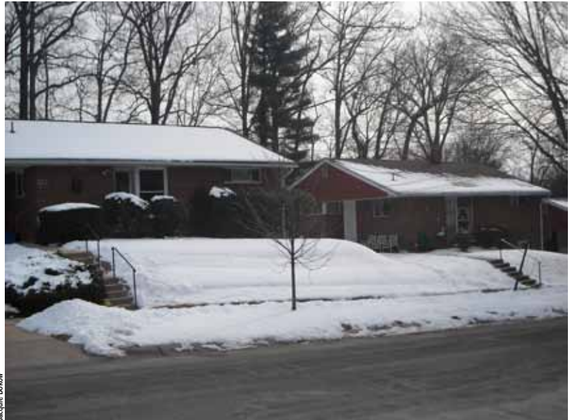
Side-by-side houses show the value of attic insulation. The unmelted snow on the house at left shows it is well insulated. The house at right has insufficient insulation in the attic so heat escapes and melts the snow much more quickly.
