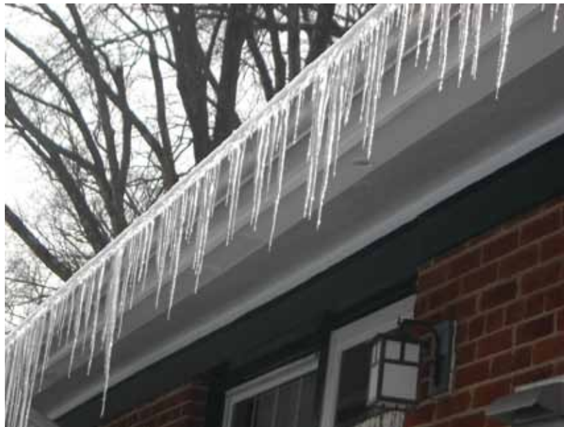
Icicles hanging from the eaves indicate heat is escaping into the attic, enough to melt the snow. Low temperatures mean the snow melt freezes again once it leaves the warmer roof.
