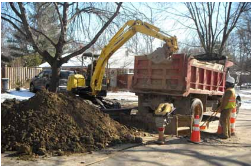
Workers for WSSC subcontractor Curt & Sons (Mt. Airy, Md.), spent days in freezing temperatures replacing sewer pipes.
